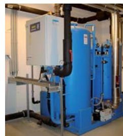
Absorptionskältemaschine 30 kW Solution / EAW
